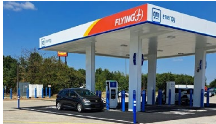
EV Charging Stations
